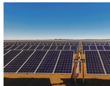
Power Plant Kimberly Droogfontein South Africa System Capacity: 250 MW
