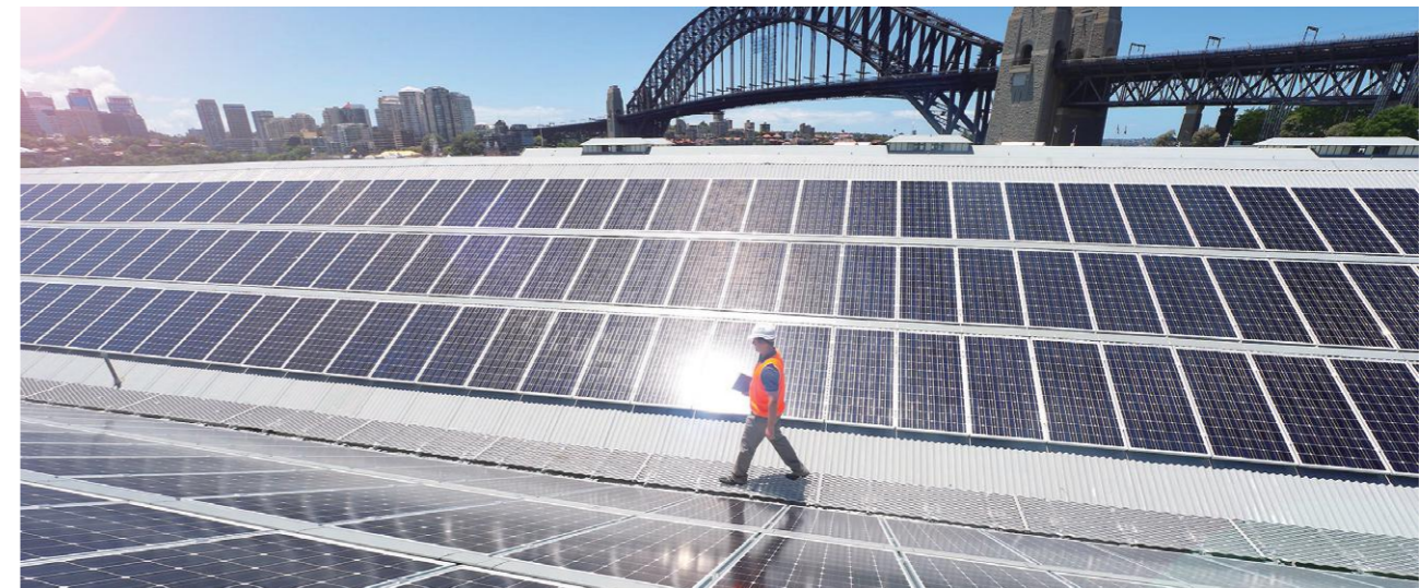
Sydney Opera House Rooftop Project Australia System Capacity: 384 KW
