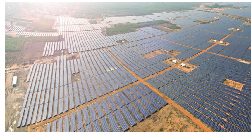
Tamil Nadu Power Plant India System Capacity: 222.5 MW
